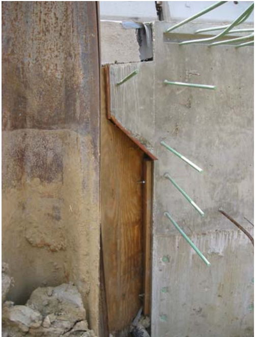
Inclined paving notch observed during construction of a new bridge
