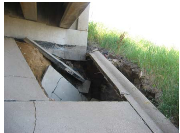
Failure of concrete slope protection due to erosion
