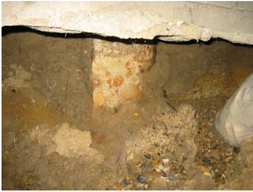
Exposed H-pile caused by soil erosion under the abutment
