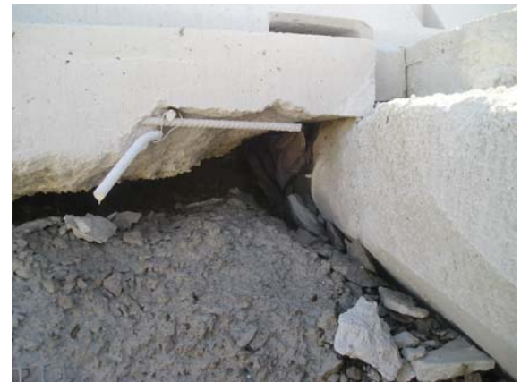
A 9-inch void under the approach slab and spalling of concrete from the paving notch and the approach slab
