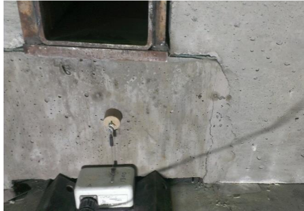
a) Propagation of crack
