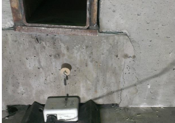
a) Propagation of crack
