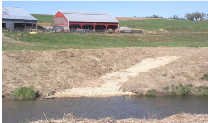
A newly installed cattle approach on the Deppe property gives livestock access to the stream at one point.
