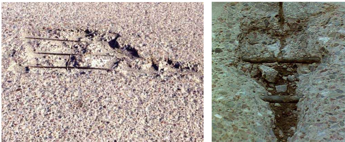
Figure 3. Corrosion of high steel (left photo) and of embedded dowel bars (right photo)
