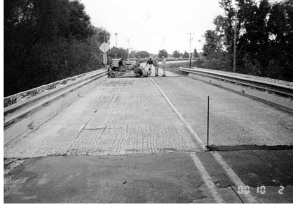
The Independence bridge after removal of unsound concrete from both lanes. Note that the majority of reinforcing steel remains covered with concrete.
