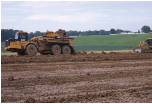
Placement of unsuitable fill
