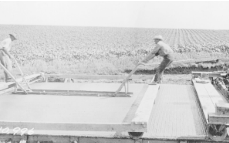
Workers using an early concrete pavement finisher, circa 1920s. Photo courtesy of Iowa Concrete Paving Association.
