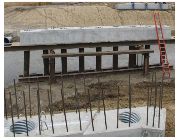
Precast abutment and pier cap in place at the Boone County bridge site
