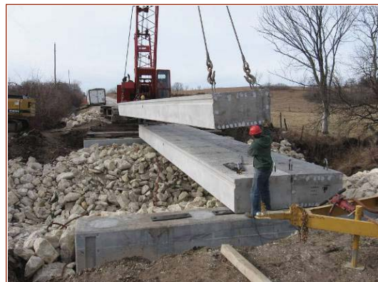
Placement of a precast box girder at the Madison County bridge site
