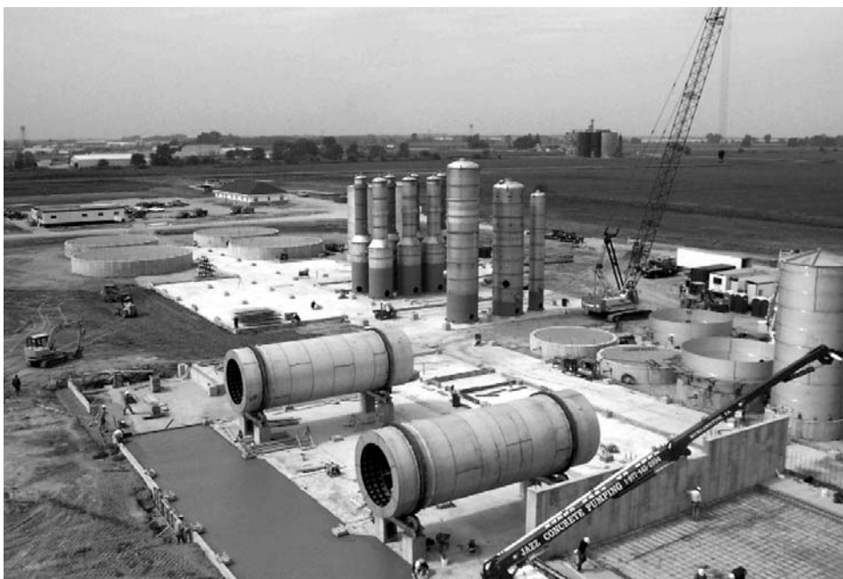
Construction is well under way on the $55 million ethanol plant of Big River Resources near West Burlington. The operation will employ 32 people and purchase 15 million bushels of corn annually.
